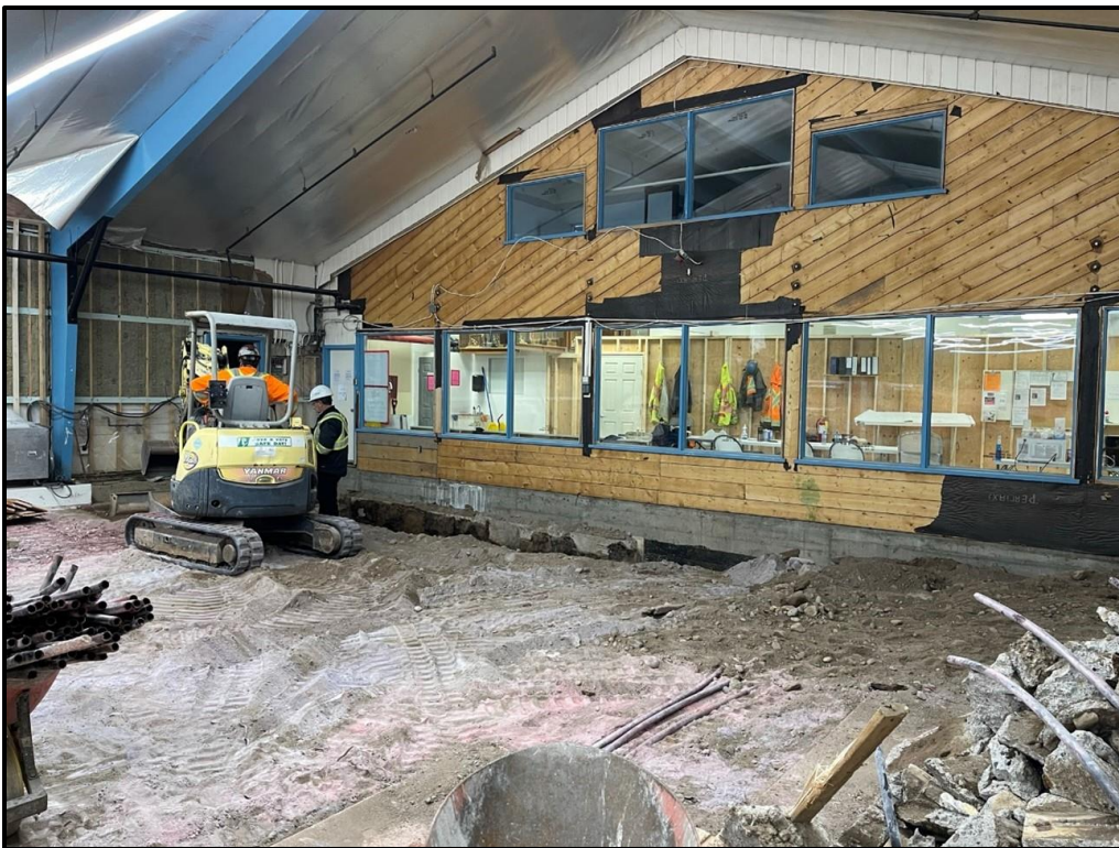
Construction works underway in the exciting upgrades to the curling club, skating rink and community hall complex
