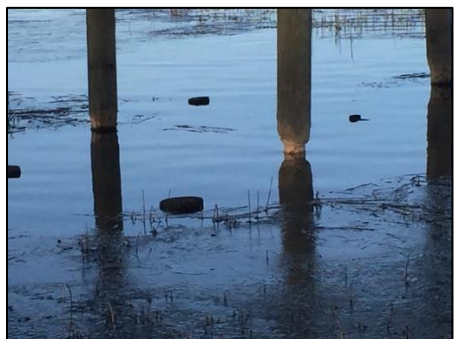
Image 1: Damage to pilings
